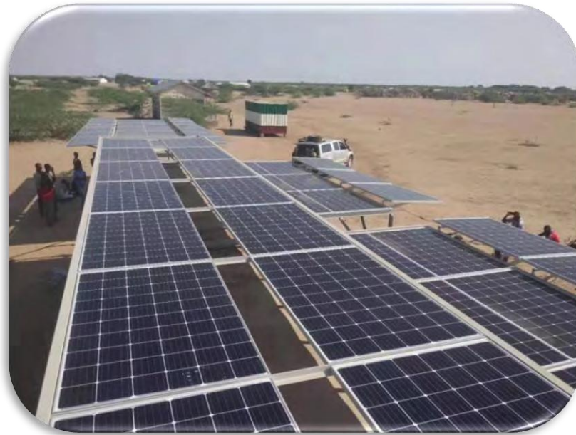
1MW Solar Power PV Station Kenya year 2015
