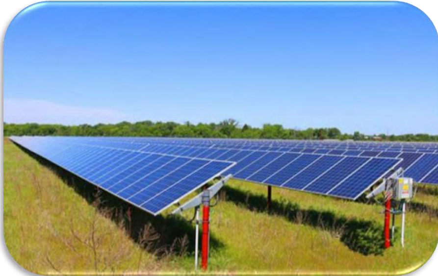
2MW Solar Power PV Station Burundi year 2018
