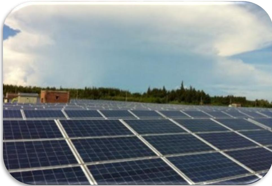
2MW On-grid Solar Power Project Malaysia year 2014
