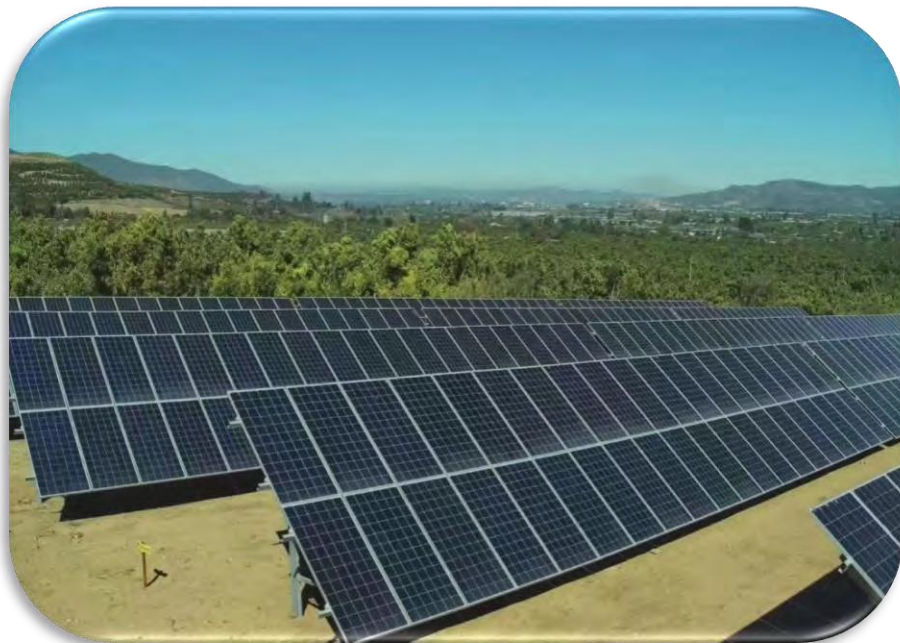
2MW Power Plant Thailand year 2012
