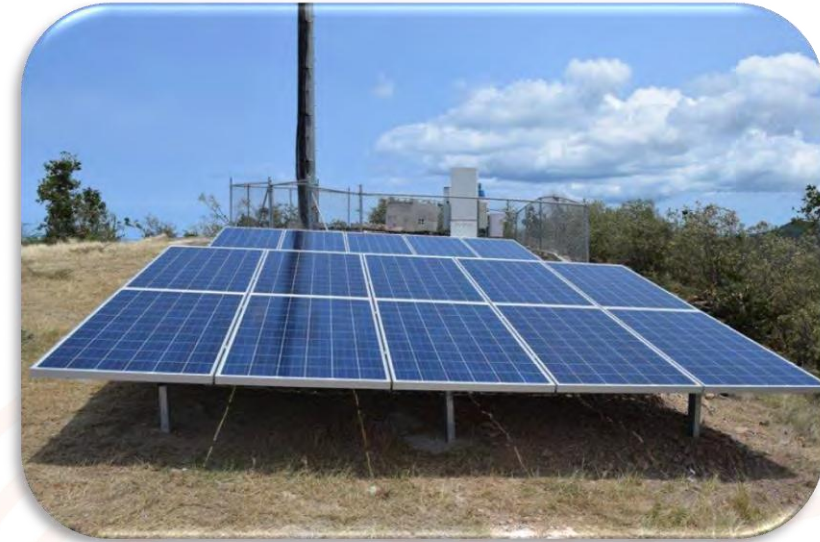
200KW Solar System Antigua 2017
