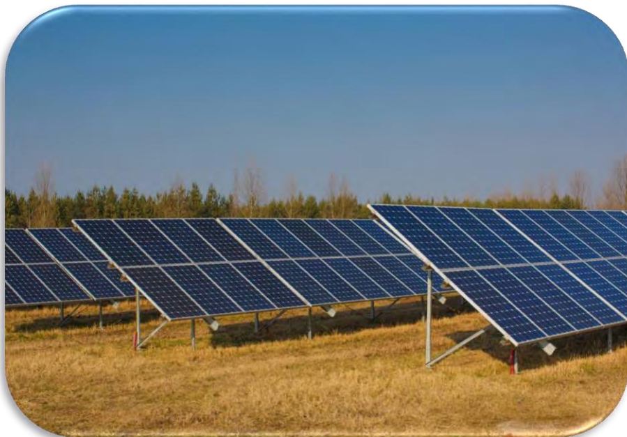
3.5MW Solar Power PV Station Czech year 2016
