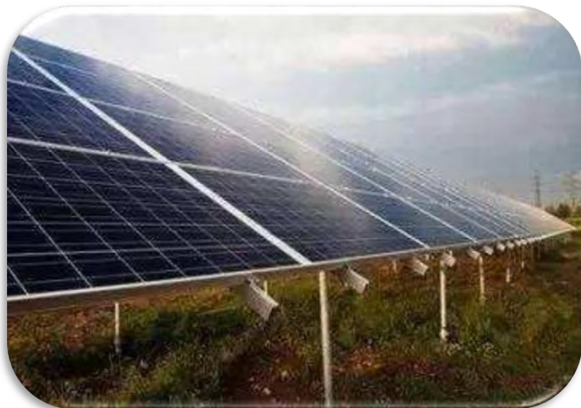
5MW Power Plant France year 2012
