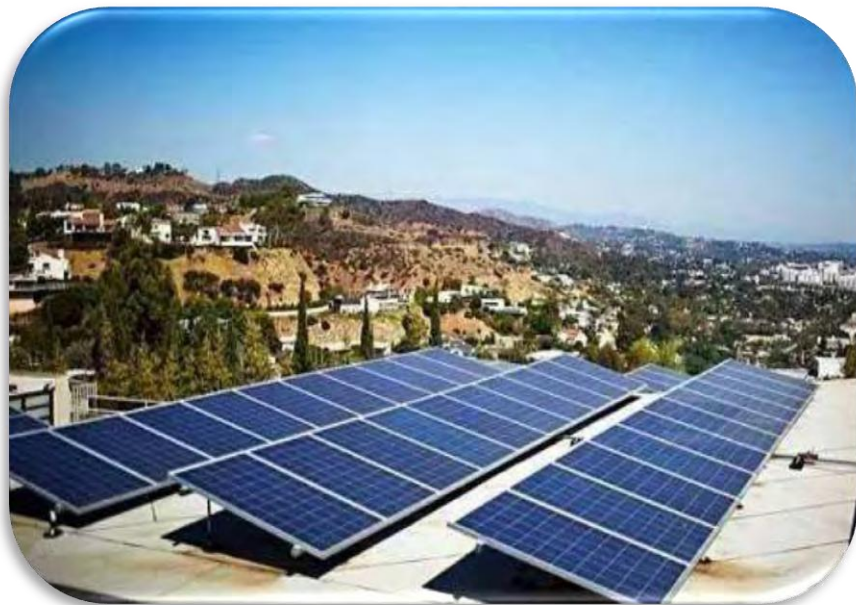
500kw Power Plant Egypt year 2017
