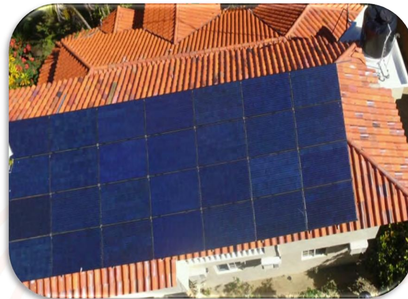
500KW Solar Power PV Station Dominica year 2016
