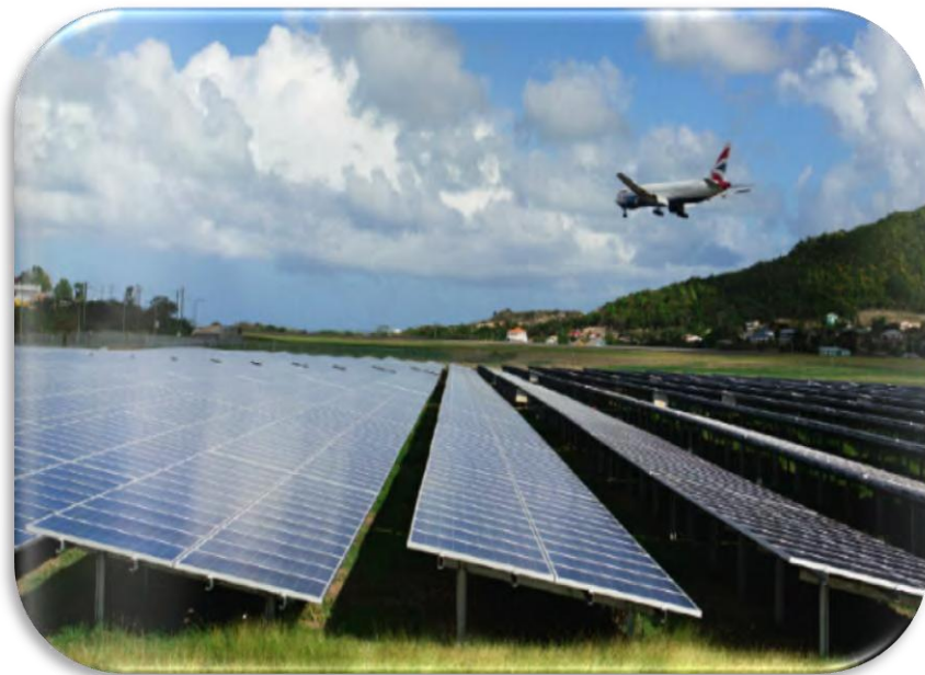
3MW Solar Power PV Station Antigua year 2016
