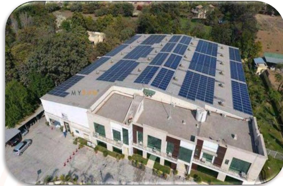
600kw Roof System Colombia year 2016
