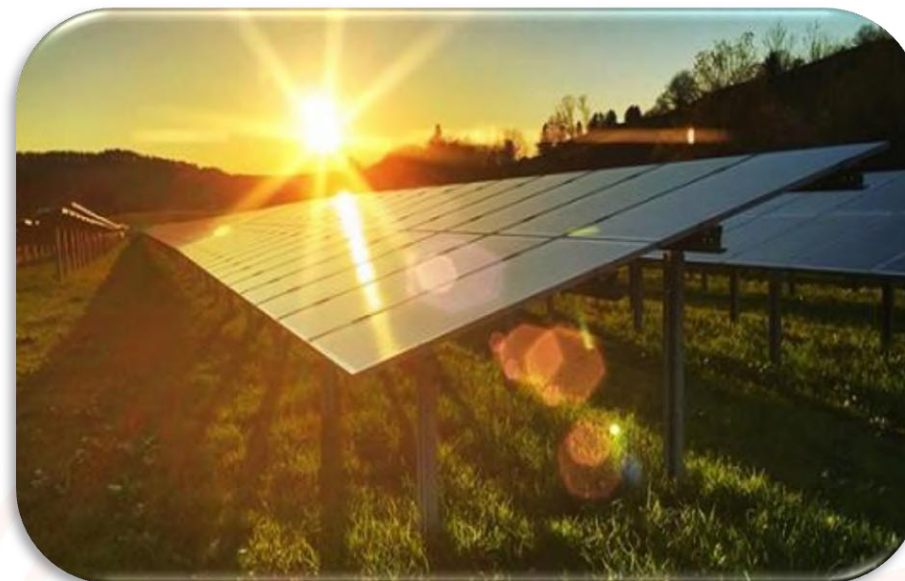
600KW Solar System Guyana 2018
