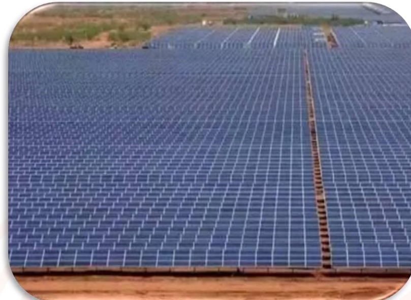
30.6 MW On-grid Solar Power Project India year 2016
