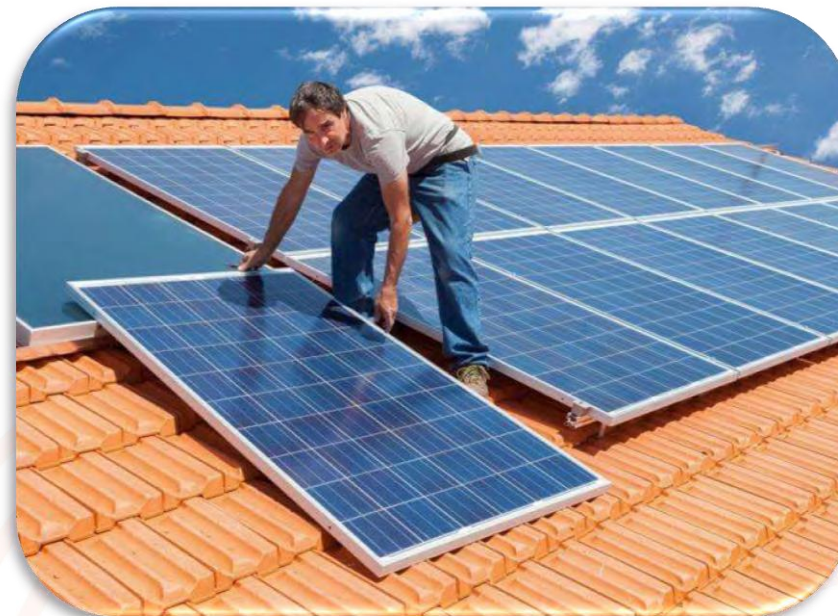
800kw Roof System Netherlands year 2014
