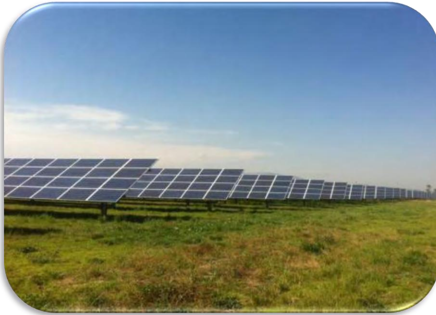
20MW Power Plant Mexico year 2017
