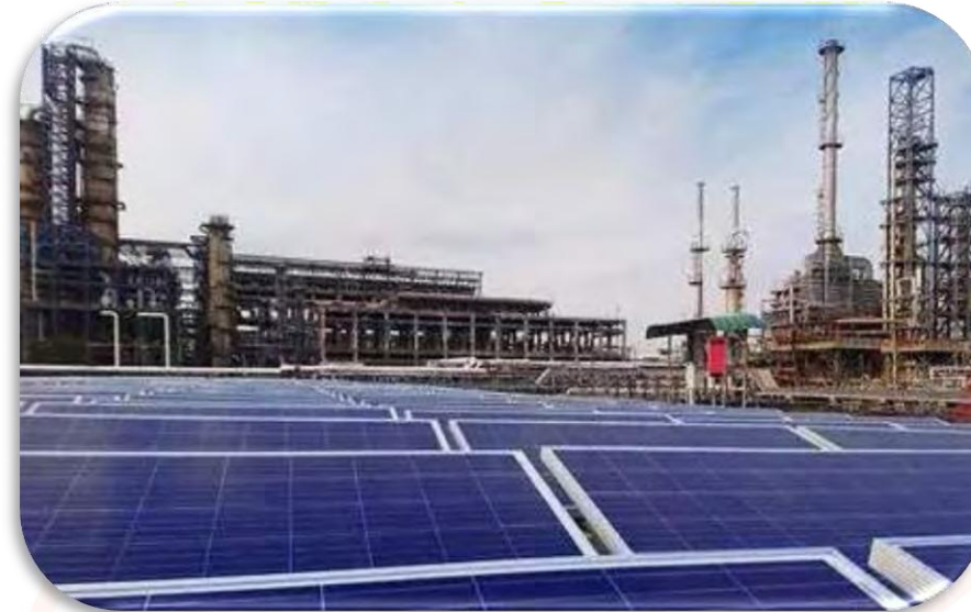
5MW Power Plant India year 2018
