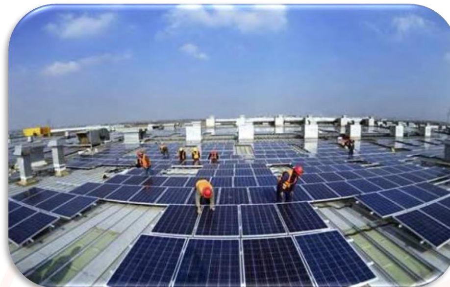
2MW Power Plant Portugal year 2018
