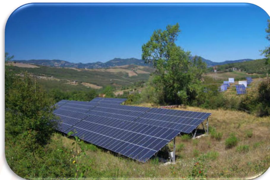
500kw Power Plant Italy year 2018
