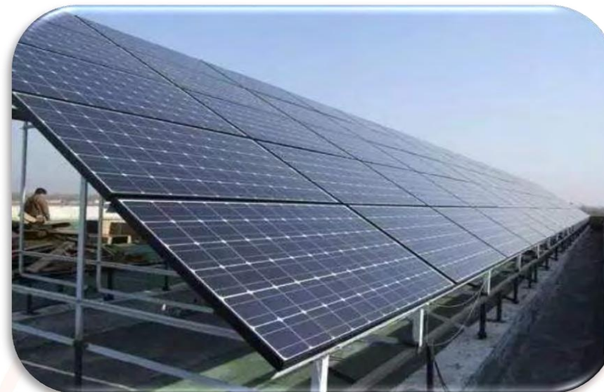
1.5MW Power Plant UK year 2018
