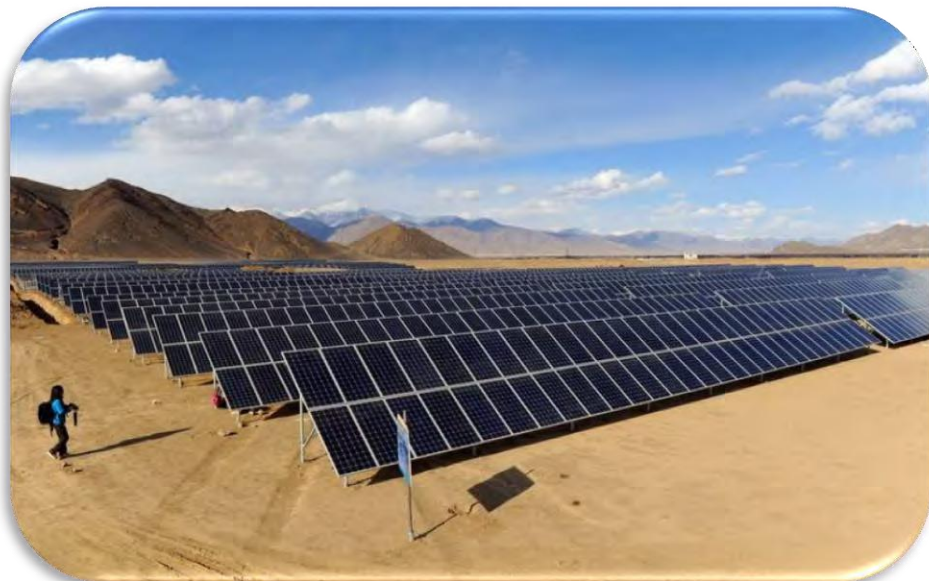
15MW Power Plant Brazil year 2017
