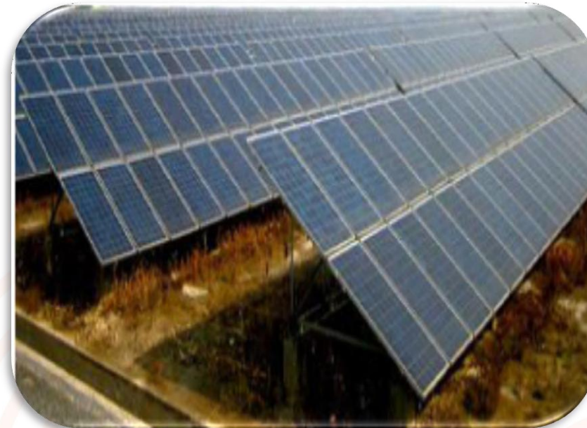
5MW Solar Power PV Station South Africa year 2016
