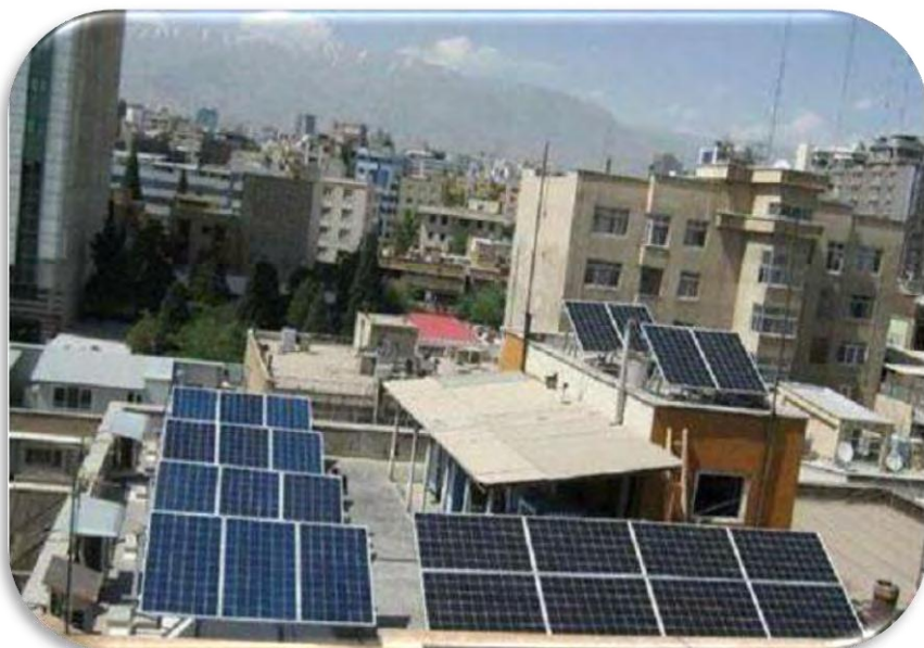
300kw roof system Iran year 2015
