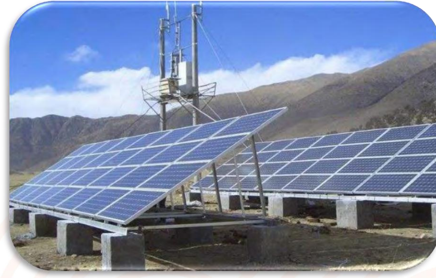
800KW Solar Power PV Station Zimbabwe year 2015
