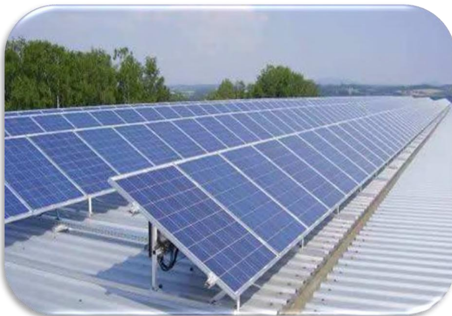
3MW Solar Power Plant Hungary year 2019
