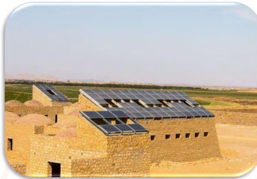
200kw Solar System Morocco year 2018
