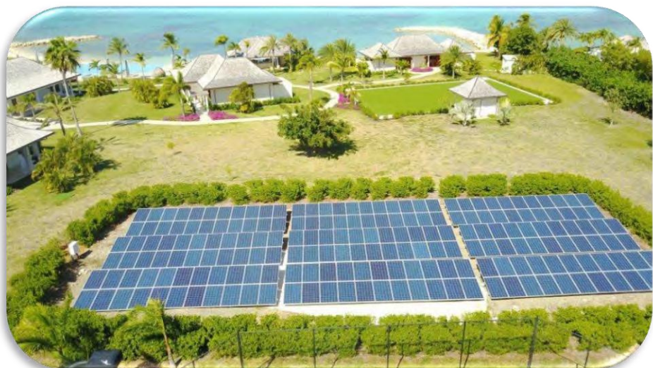
200kw Solar System Jumby Bay Island year 2017
