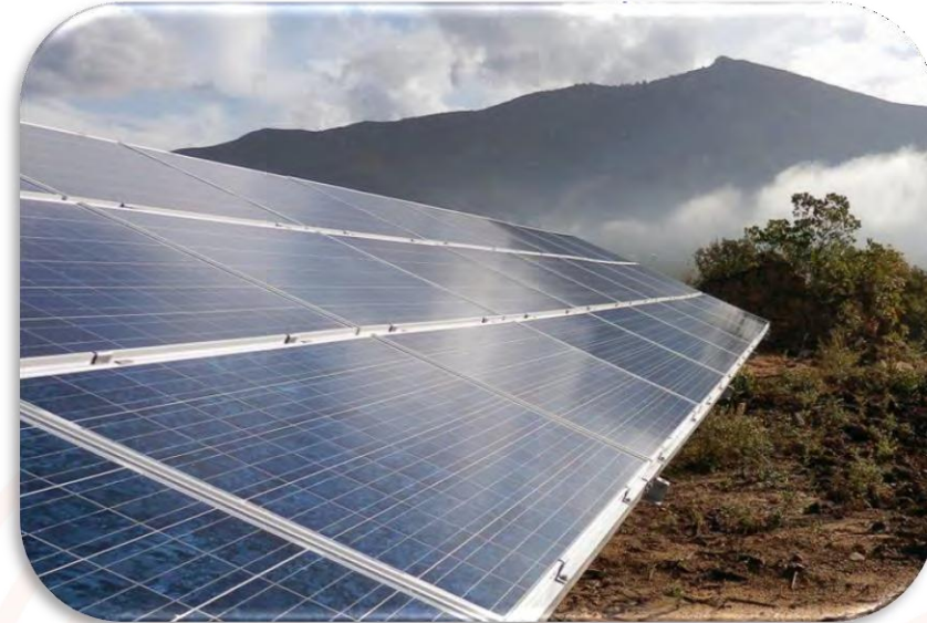
4.5MW Solar Power PV Station Corsica 2014
